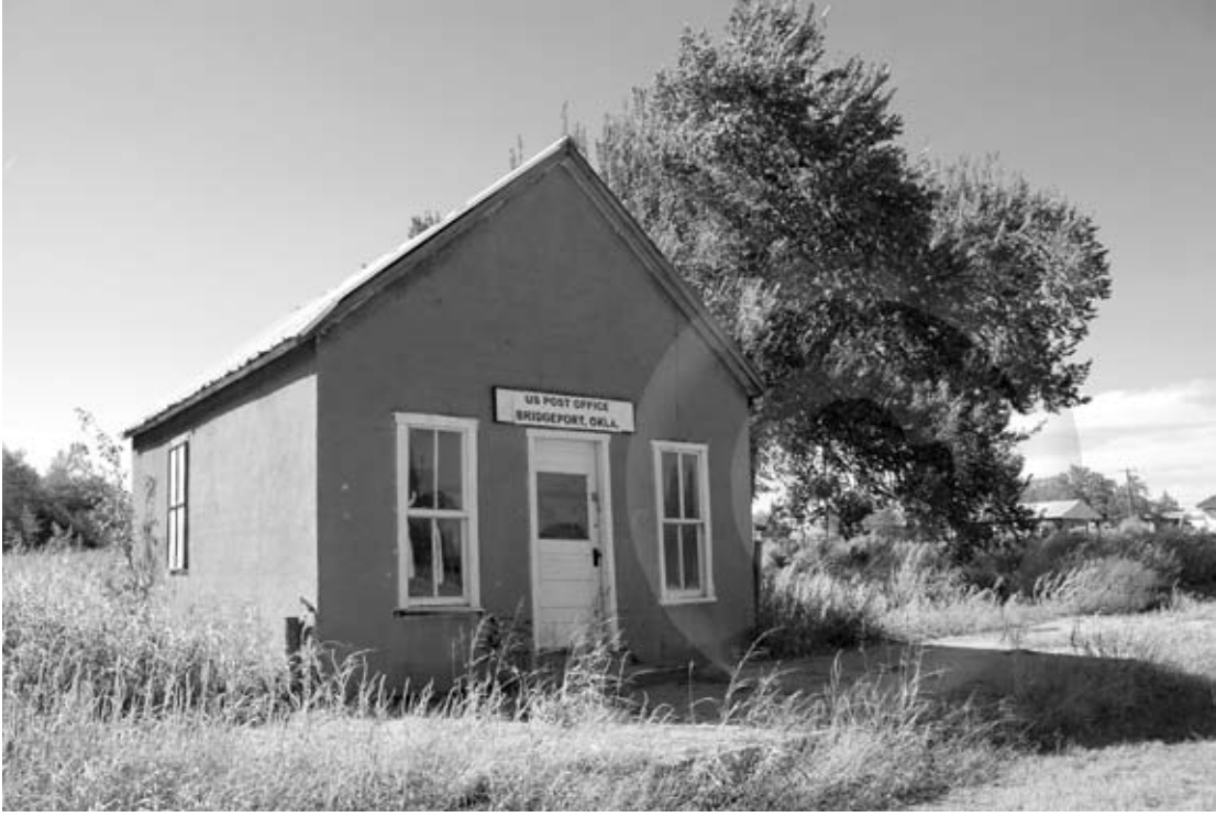
SEEN BETTER DAYS - The Bridgeport, Oklahoma post office stands alone in what was once the bustling business district of the Caddo County town.
